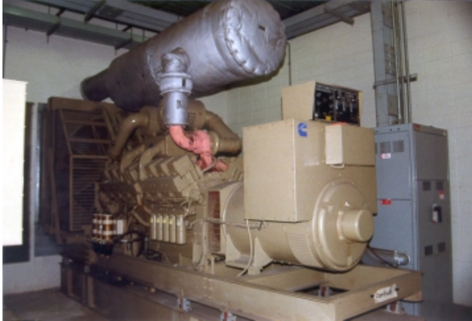
Figure 11-4. Diesel-powered backup generator
