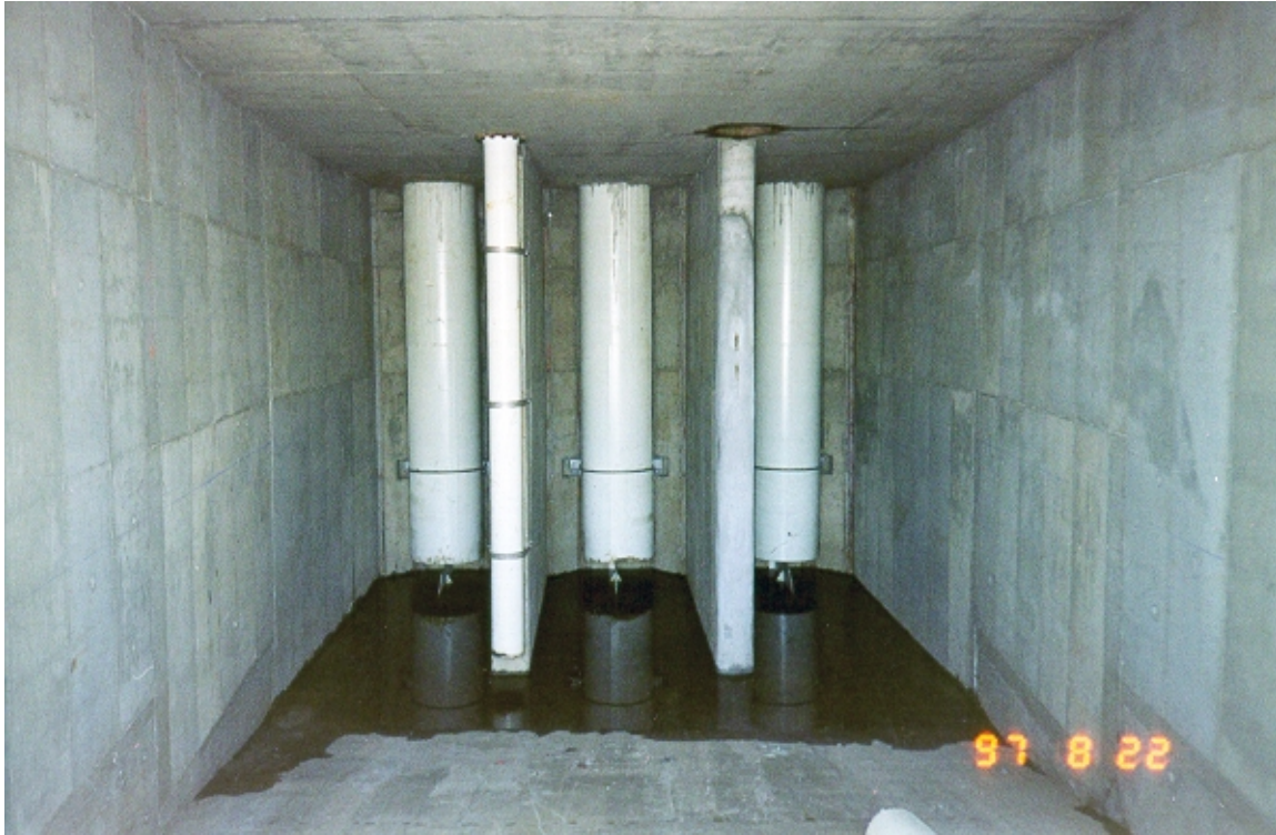
Figure 3-10. Rectangular pit with submersible pumps
