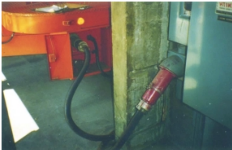
Figure 11-5. Mobile generator and standby power receptacle
