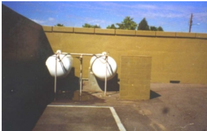
Figure 11-1. Liquid propane tanks for pump station power
