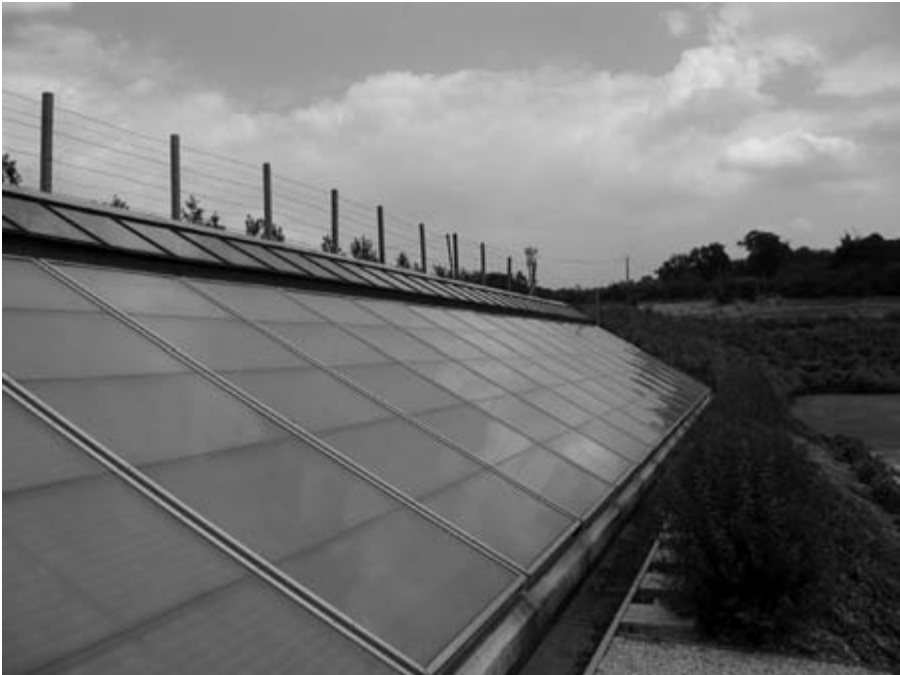
Solar Array, RES Group Head Office – Beaufort Court, Hertfordshire, England Hybrid thermal/photovoltaic solar energy panels. The system produces electrical energy and hot water [RES]
